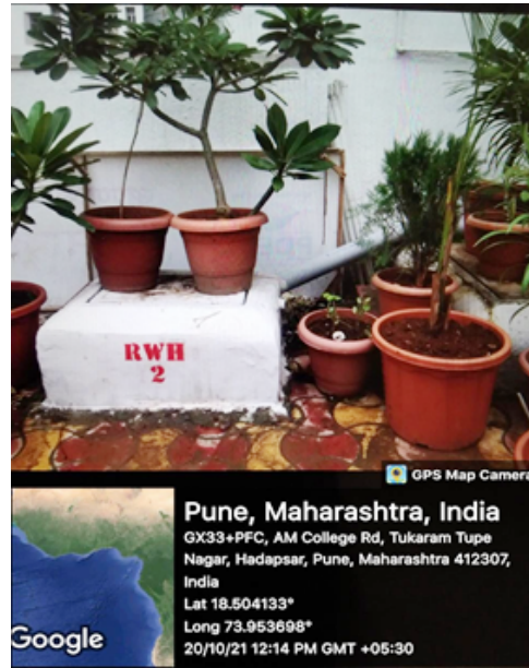
Rain harvesting unit 2
