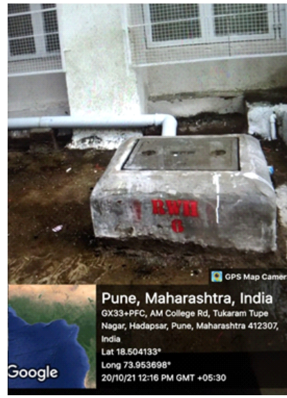
Rain harvesting unit 6
